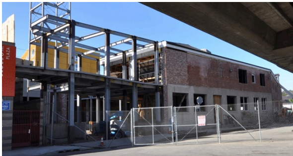
Figure 7: Capitol Milling Company building, view of east elevation from N. Spring Street (GPA, 2018)
